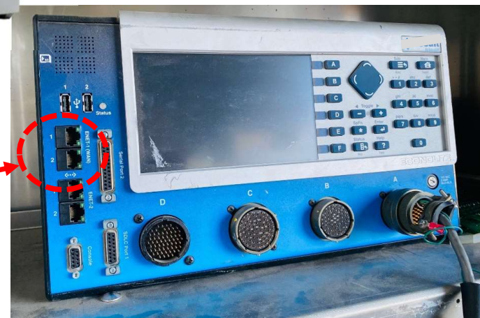
TS-2 Type 2 Controllers With Ethernet Port that serves to connect to fiber
